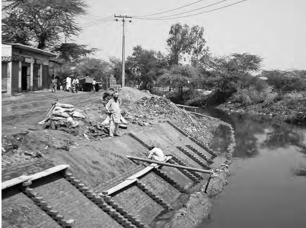
Photo 6.3: The retrofitting of a lining of local bricks along a drainage ditch in Lahore Pakistan. Accumulated debris, sediment and vegetation has been removed from the ditch, the bank re-profiled. Source: Peter Lingwood.
