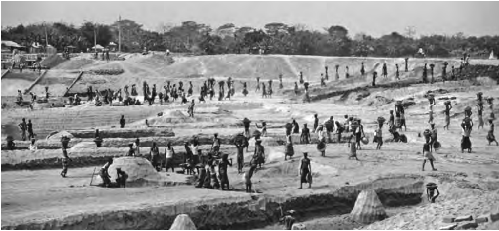
Photo 3.4: Labor intensive construction of river flood protection embankments in Bangladesh. Source: Alan Bird
