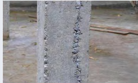
Figure 3.5 “Honeycombing” showing shoddy construction
