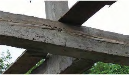
Figure 3.4 Debris embedded in a concrete support beam
