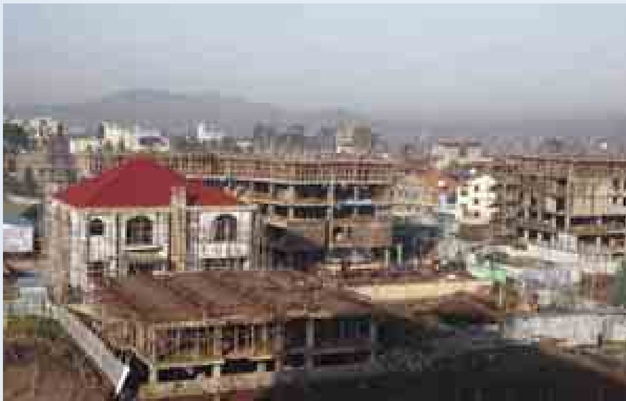
▲ New buildings are constructed in Addis Ababa, Ethiopia. Situated in the foothills of the Entoto Mountains and standing 2,400 metres above sea level, Addis Ababa is the third highest capital in the world. The city has a population of about two million.
