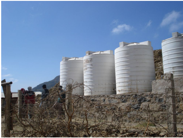
Figure 9: There are five 3000 liter tanks for fog water at Arberobue, Eritrea (2007).
